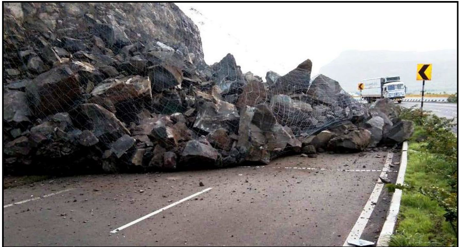
Fig. 9 Landslide occurrence at P11 site on July 14, 2019
